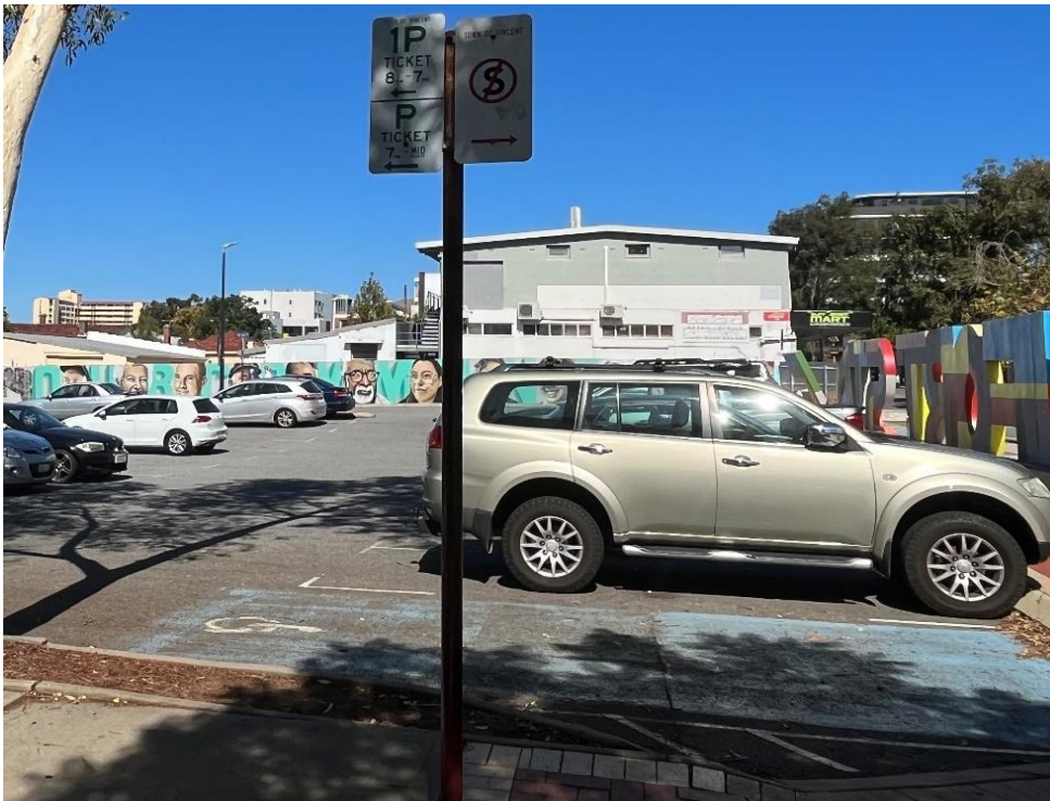
Figure 6.6 Non-compliant ACROD parking bay at Barlee Street
