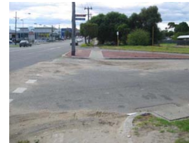
Figure 5: Poor pedestrian crossing across Jugan Street
