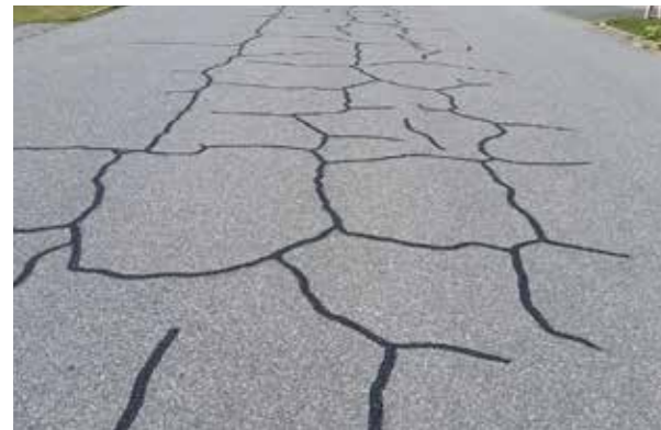
An interim crack sealing, - preventative maintenance, to extend the life of the asset (Fleet St – Access Road)
