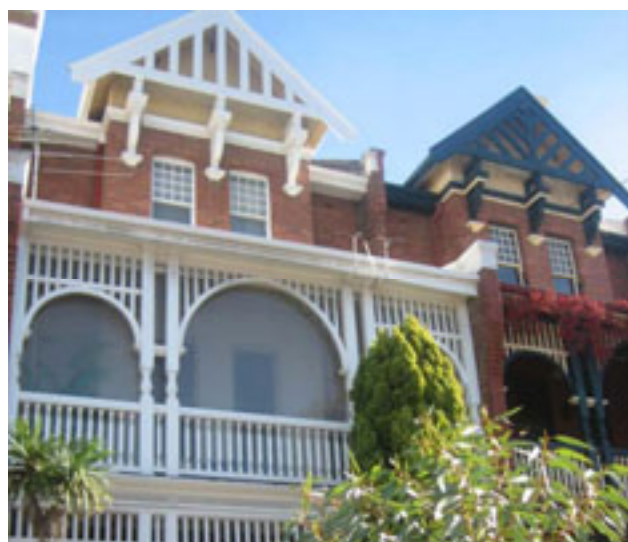
Owners of one of the Federation Filigree Beaufort Street Terraces were provided with funding for the removal of paint work on the ground storey façade and for re-tuck-pointing.
