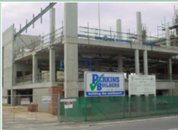
The new Department of Sport and Recreation's office building fronting Vincent Street, Leederville, takes shape.
