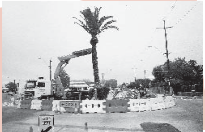
Traffic Management: A Canary Island date palm being lowered into place in the centre of the new roundabout which replaced traffic lights at the intersection of Bulwer, Smith and Brisbane Streets, Perth.
