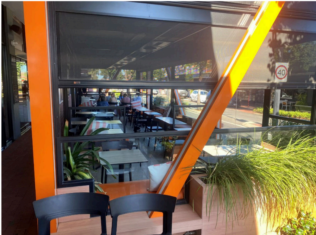
Figure 2 – Alfresco Structure as viewed from the west with a section of the woven mesh blinds in use
